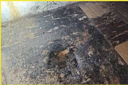
1.3 Dripping in basement
