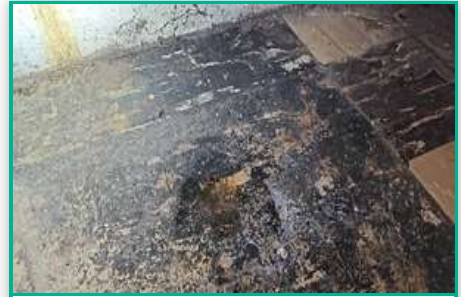
1.3 Dripping in basement
