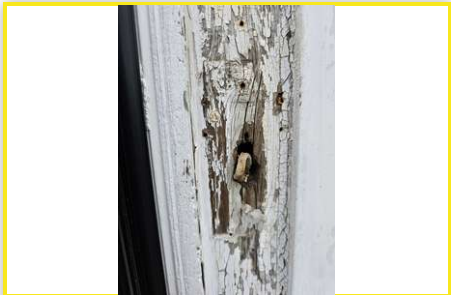
1.1 There used to be a doorbell here
