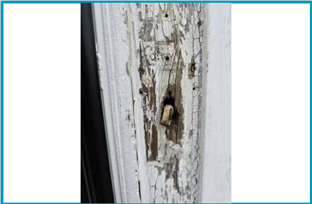
1.1 There used to be a doorbell here
